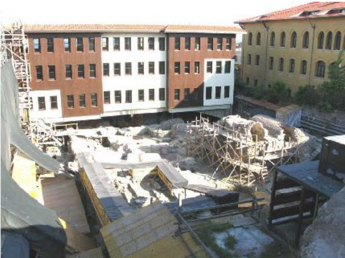
Above: the first structure of the three proposed extensions currently under construction in front of the present hotel, the former Sultanahmet prison (the yellow-painted building in the right).
