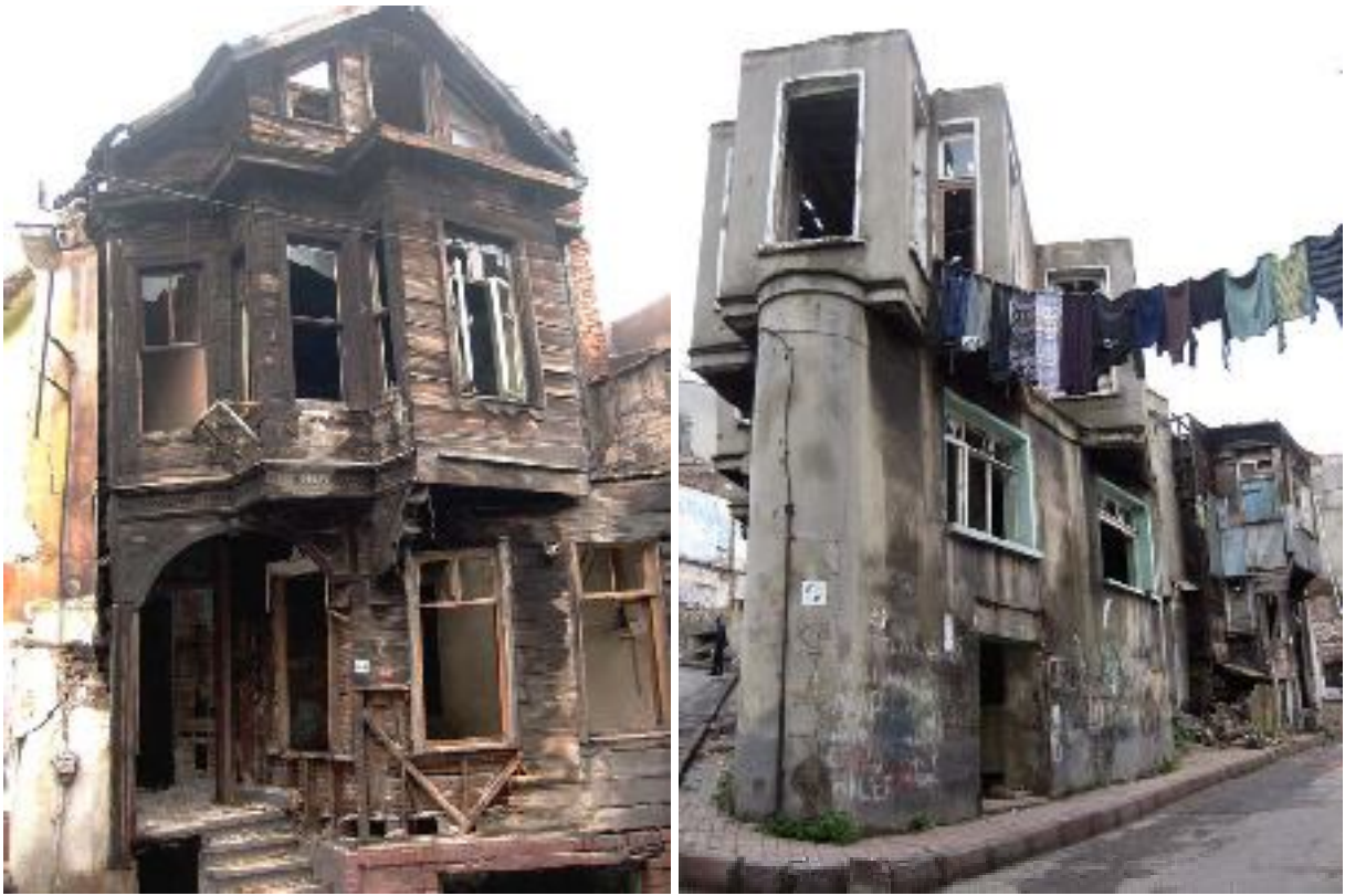
Above: two of the nine historic listed houses illegally demolished by KIPTAŞ on 18 th November 2007.
