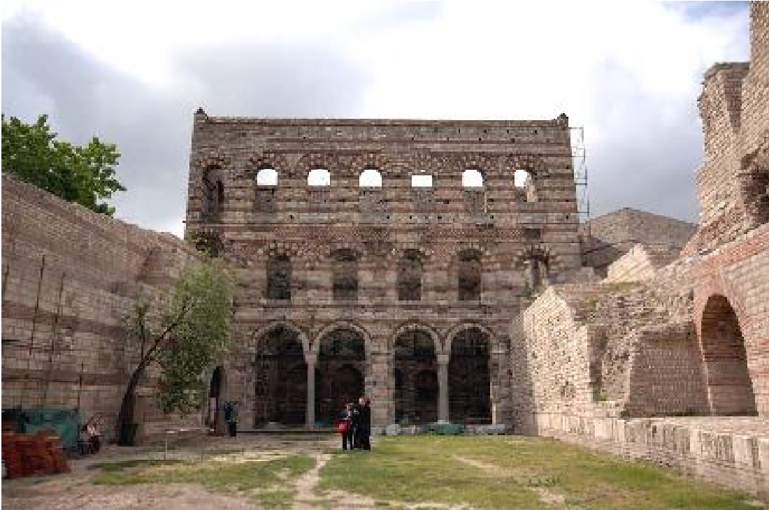
Above: Tekfur Saray, a Byzantine palace building. Work carried out to the adjacent walls since the 2006 mission involved excessive replacement of facing stones and bricks and the creation of new flat wall tops.
