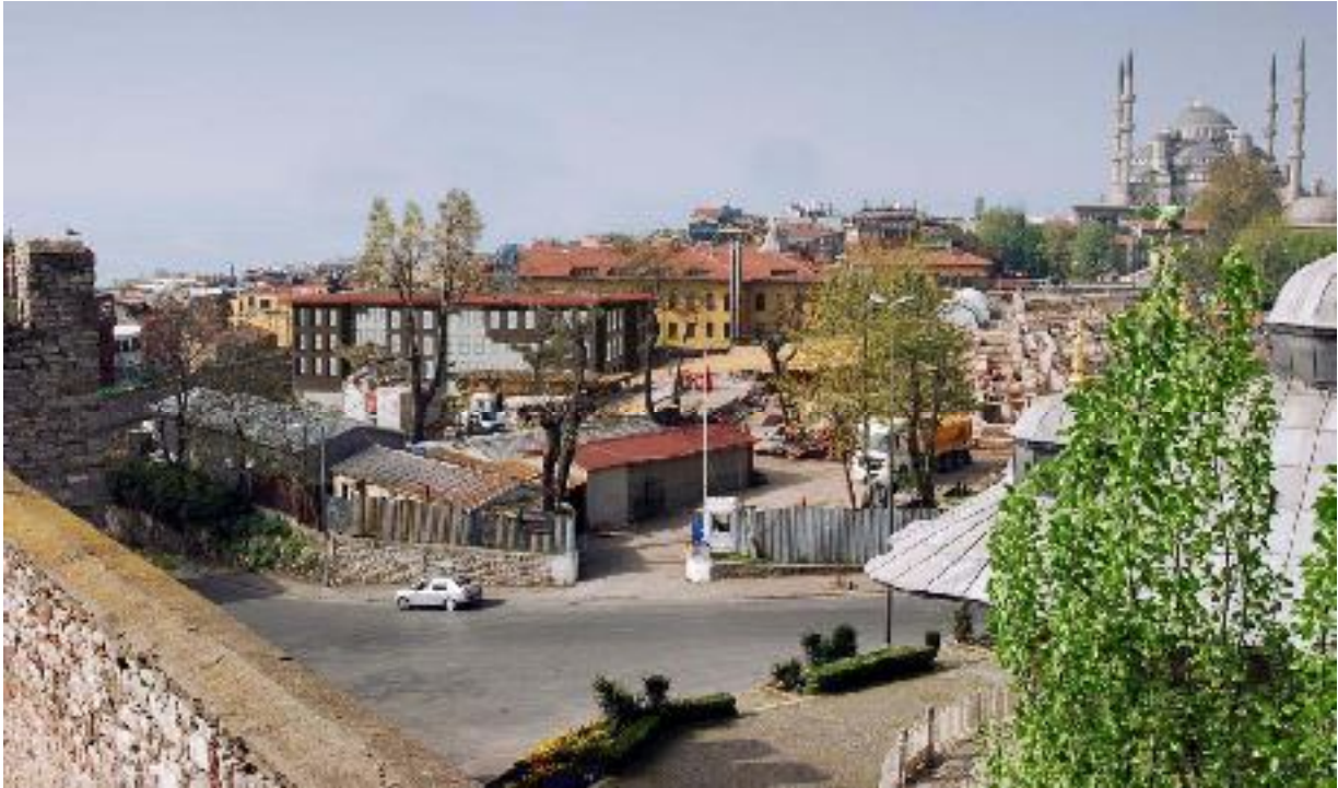
Above: the extensions currently under construction in front of the present hotel, the former Sultanahmet prison (the yellow-painted building in the centre). In the background is the Blue Mosque, in the foreground the Ahmet III Fountain and the walls of Topkapı Palace.
